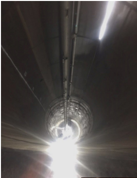
Inside A Digester from 4th floor
